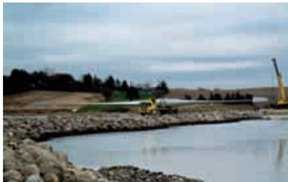
6 When installing the N60/1300 kW machine under normal conditions, the hub is installed together with the nacelle, and the blades are mounted individually to the hub. At Ebeltoft blades were mounted to the hub on shore. Thereafter, they were transported to the turbines at the pier.
