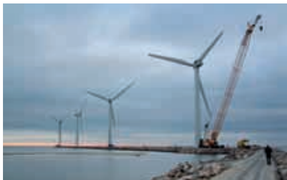
8 The turbines are now erected and the transformer stations have been mounted inside the towers.
