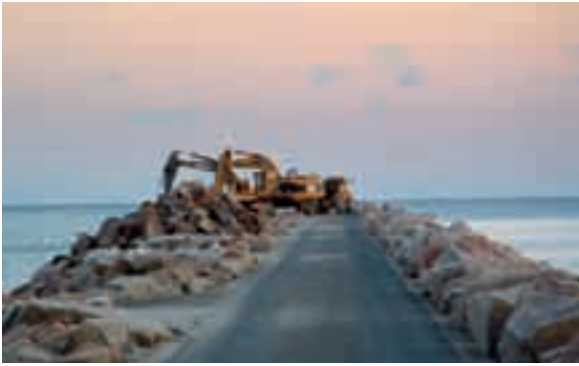
1 The old wind turbines and foundations have been removed from the pier, and the pier is now broadened for the larger Nordex turbines. The new foundations are pile foundations on the ocean bed. The cables have been laid down in the pier.
