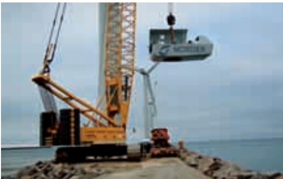
5 The nacelle is lifted to the top of the tower. From the photo it appears that the crane is too broad for the pier road. Each time the crane should start installing a new turbine on a new turbine site, it had to be dismantled.
