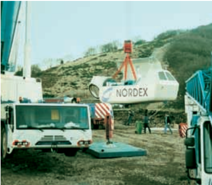
The nacelle is lifted by the crane, and then mounted to the tower.
