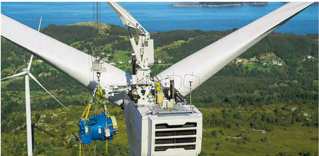
Nordex service staff replacing a gear unit using a self-hoisting crane at a wind farm in Norway.
